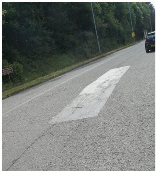
IMAGE 8 – Overbanding Example, Margam Interchange Roundabout.
