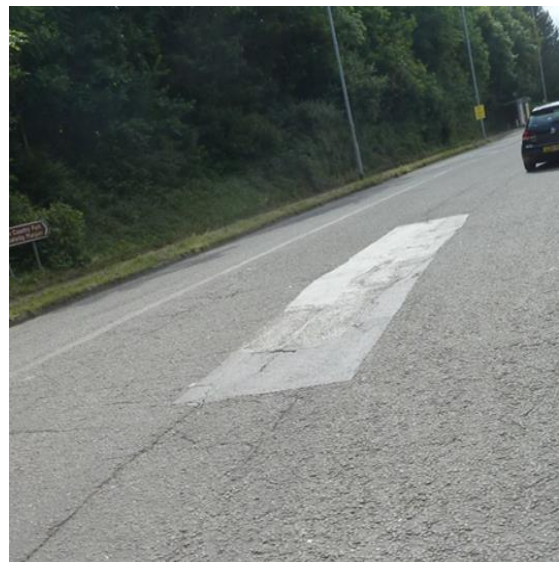
IMAGE 6 – Overbanding Example, Margam Interchange Roundabout.
